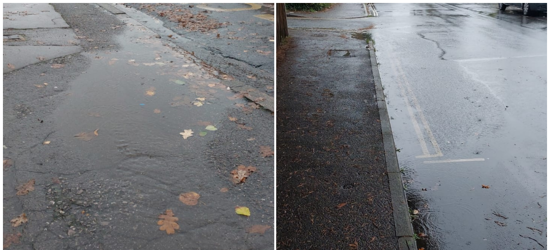
Figure 7. Examples of flooding due to degraded repair (left) and land dips (right) on Woodcote Road.
